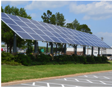
Ground-mounted solar panels.
