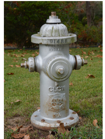
A fire hydrant.
