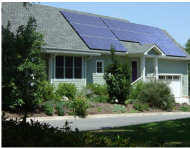
Roof mounted solar panels.
