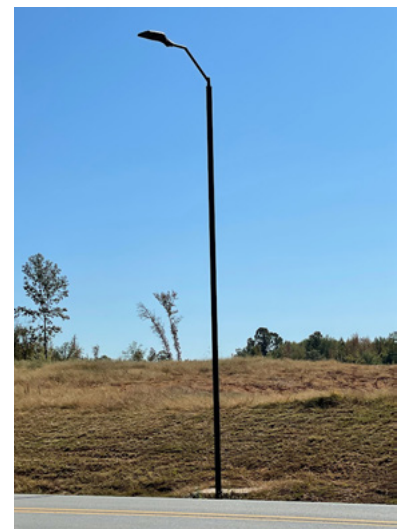
Examples of residential street lighting.
