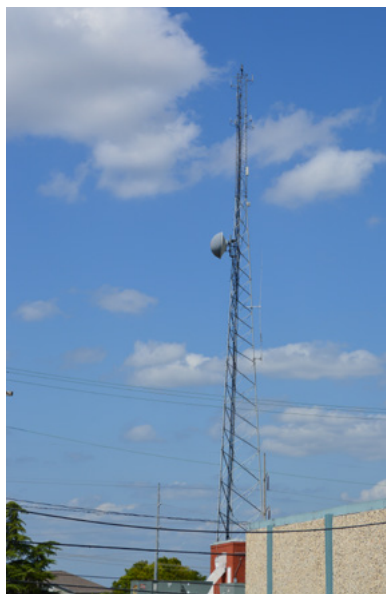
A freestanding wireless communication tower.
