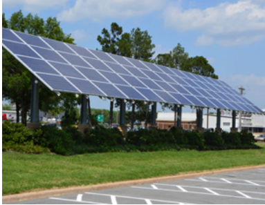
Ground-mounted solar panels.
